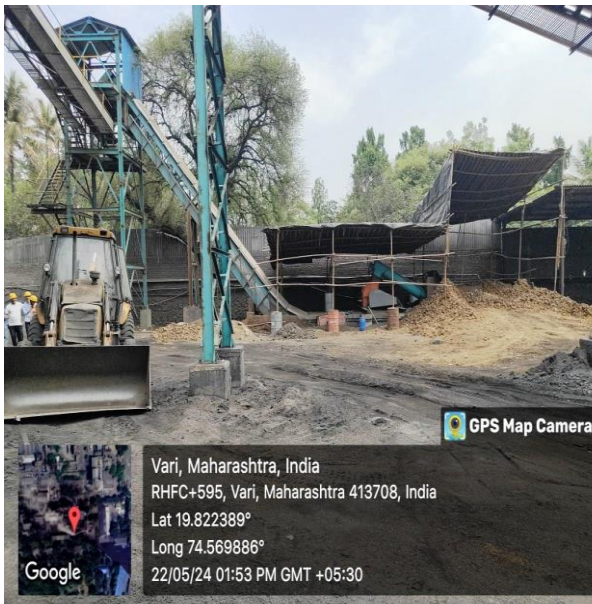
Mechanized and closed system for alternative fuel i.e. biomass shredder & feeder.
