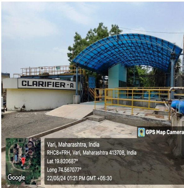
Secondary clarifier of ETP.
