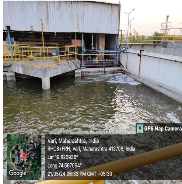
Equalization tank of ETP.
