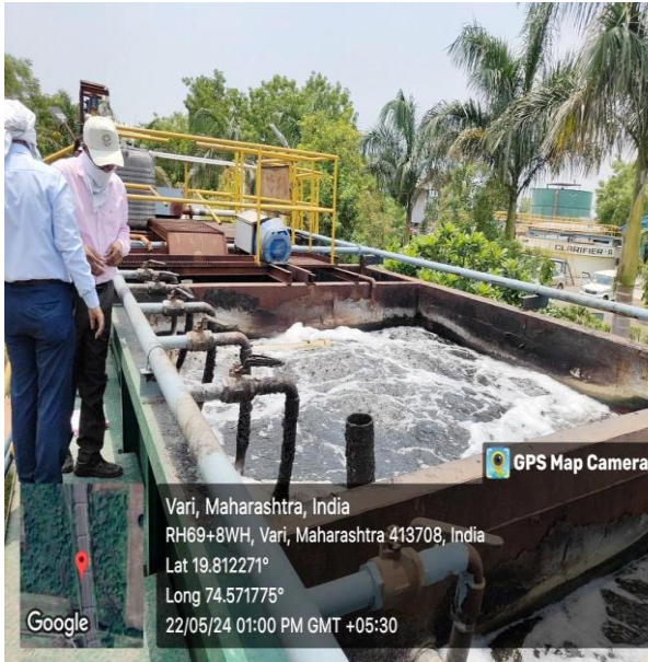
MBBR tank of STP.
