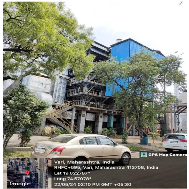
Newly commissioned 30 TPH AFBC boiler.
